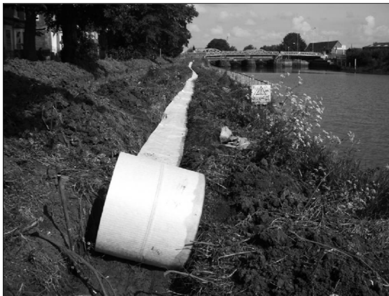
Figure 2. Fibre optic sensor cable by TenCate
